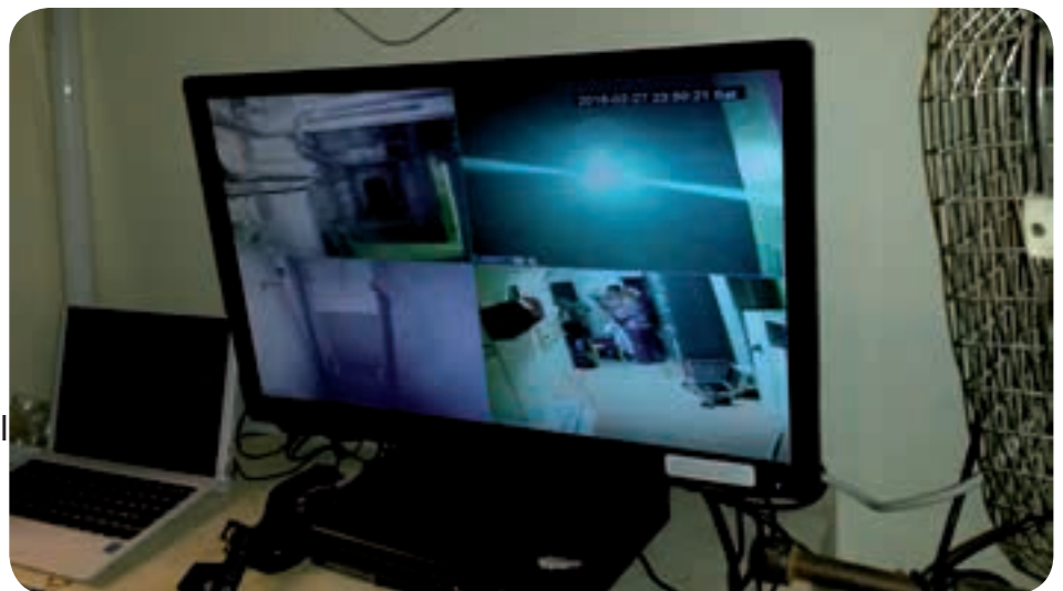
Cameras set up in various positions in the vaults
